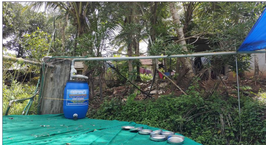
RAINWATER HARVESTING SYSTEM
